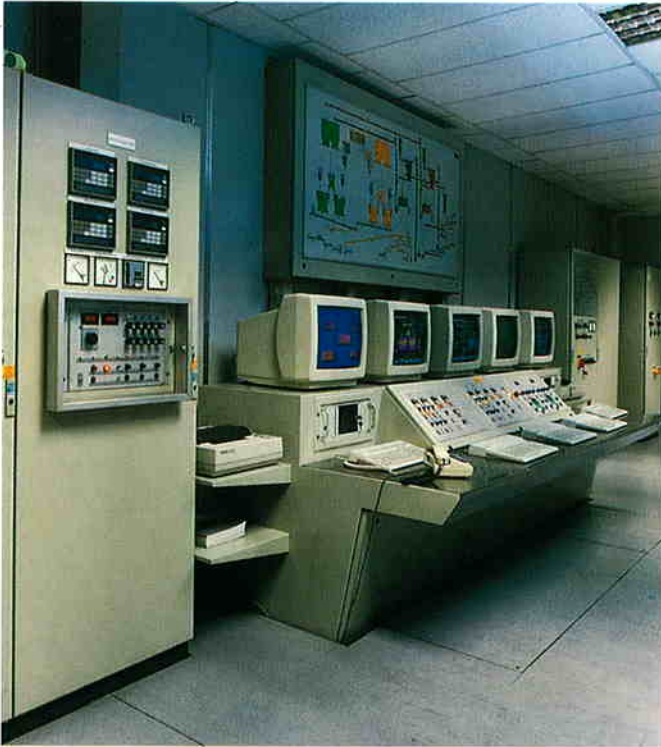
Fig. 13.1: Control room featuring CAQ system
