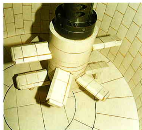
Fig.10.3: Ceramic tile lining on all surfaces
